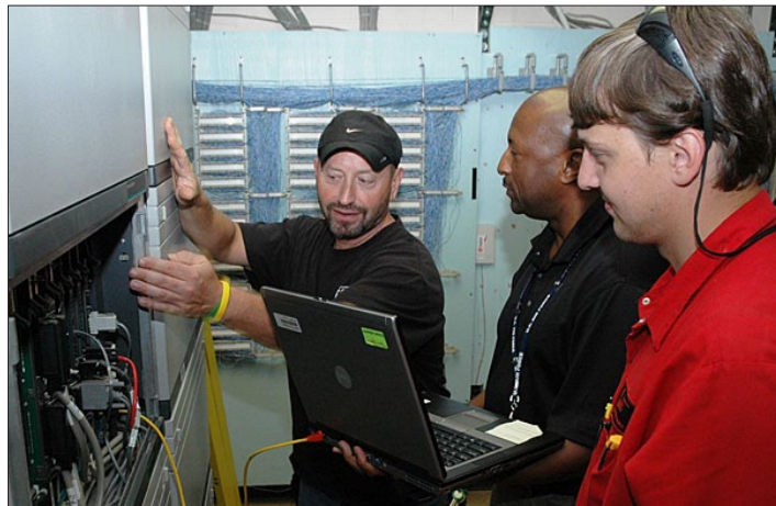
Robin DeMark John Syme and Reggie McCrimmon, Fayetteville VAMC information technology and telecommunication specialists, verify power and cabling requirements for the new phone system with Stoney Chance, electrical sub-contractor.
