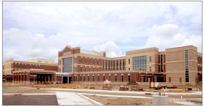
Courtesy Photo Interior finishes are nearing completion and equipment installation is underway at the Fayetteville HCC. A grand opening is tentatively scheduled for Nov. 20.
